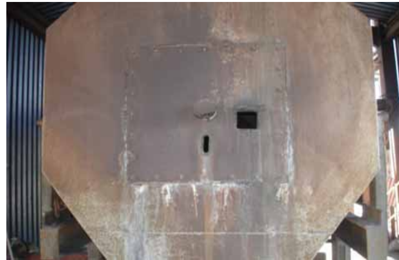
Damaged seal ring and holed discharge point
