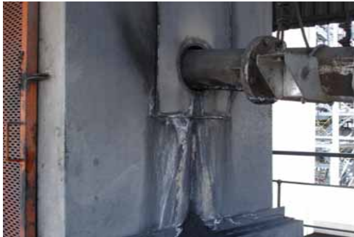
Regeneration kiln holed on feed – point without seal.
